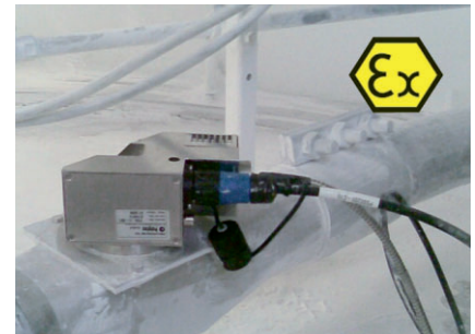
Fig. 2: Contact sensor head in potentially explosive environment.
